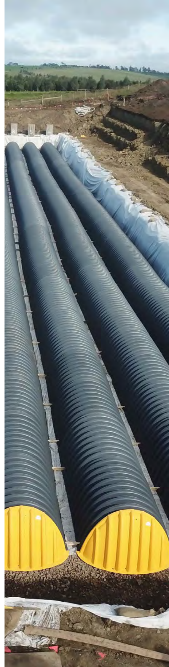
Pictured (right): The project site's 1.6 million-litre SPELChamber Detention tank for which the Baffle Box provides primary stormwater treatment.
