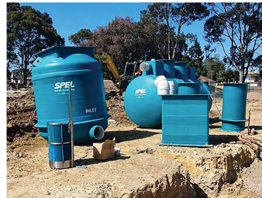
Pictured (top right): A Stormceptor installation from another SPEL project. Pictured (bottom left): A Stormceptor-Hydrosystem treatment train to be installed at another project site.
